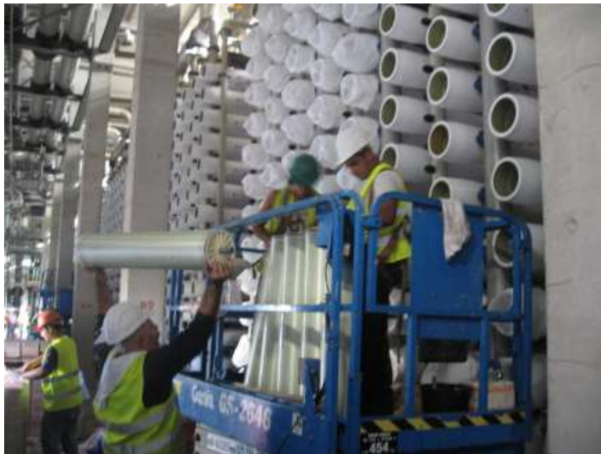
Figure 6: Hadera desalination plant
