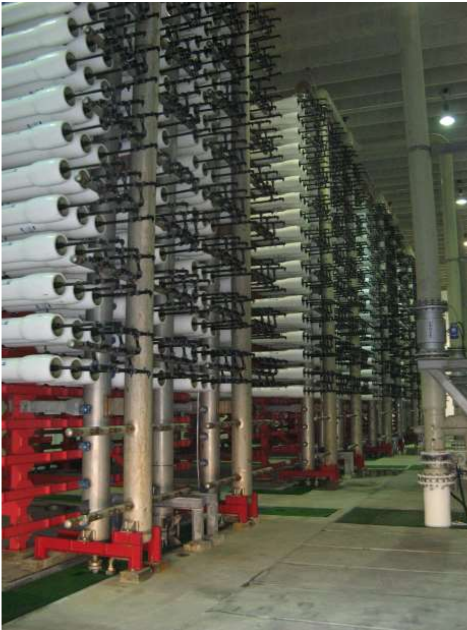
Figure 5: Palmachim desalination plant
